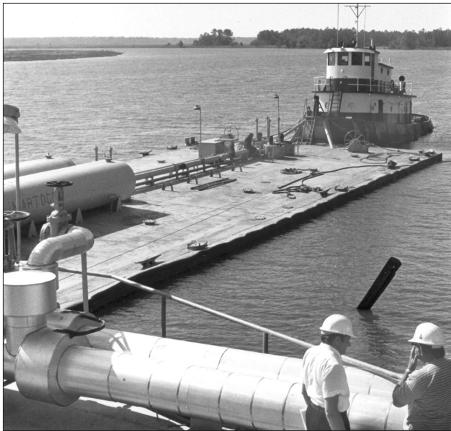
Impedance heating used to facilitate pumping of fuel oil from barges to storage tanks at power generating utility.
